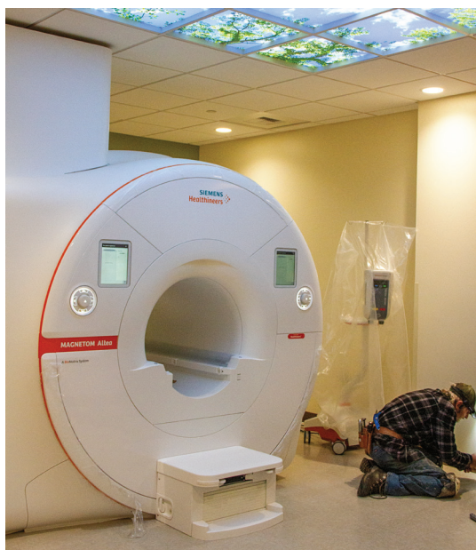
A work crew puts finishing touches in the new MRI room at St. Luke Community Hospital.
